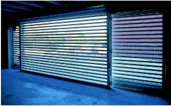
Perforated Shutter door, inside view looking out.
